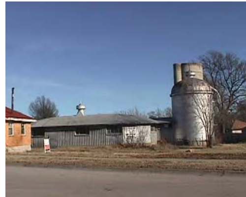
The workshop participants listed this old barn at the corner of Hutchison and Calhoun as unique asset to their neighborhood.
