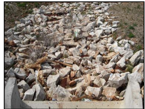
Looking downstream, below a culvert outfall, at a riprap velocity dissipation pad.
