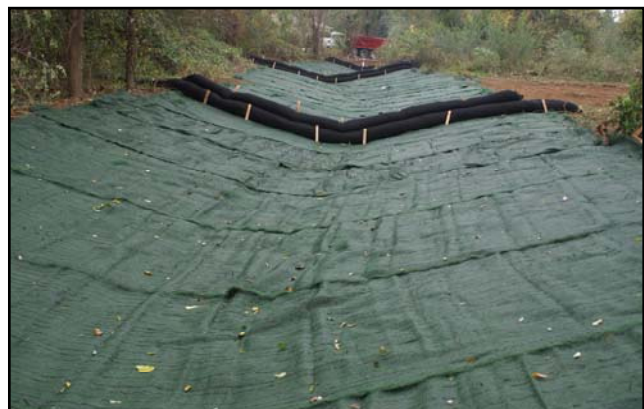
TRMs being used as a channel lining. Checks dams are in place until vegetation is established
