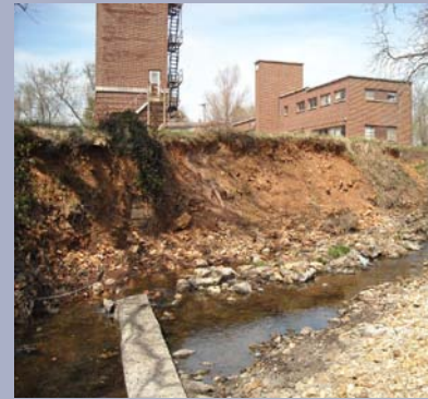
FIGURE 4: EROSION IN FASSNIGHT CREEK
