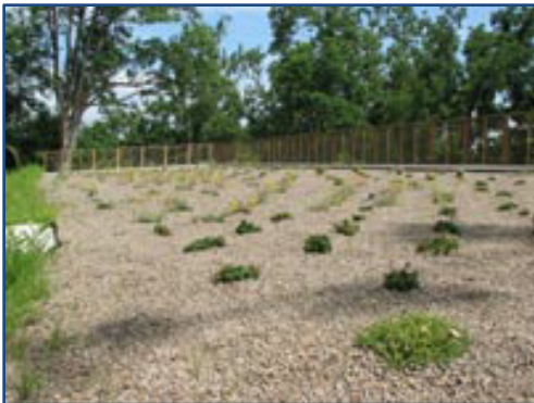
Watershed Center, 2450 E. Valley Water Mill Road: Green roof, pervious pavement, rain garden...
